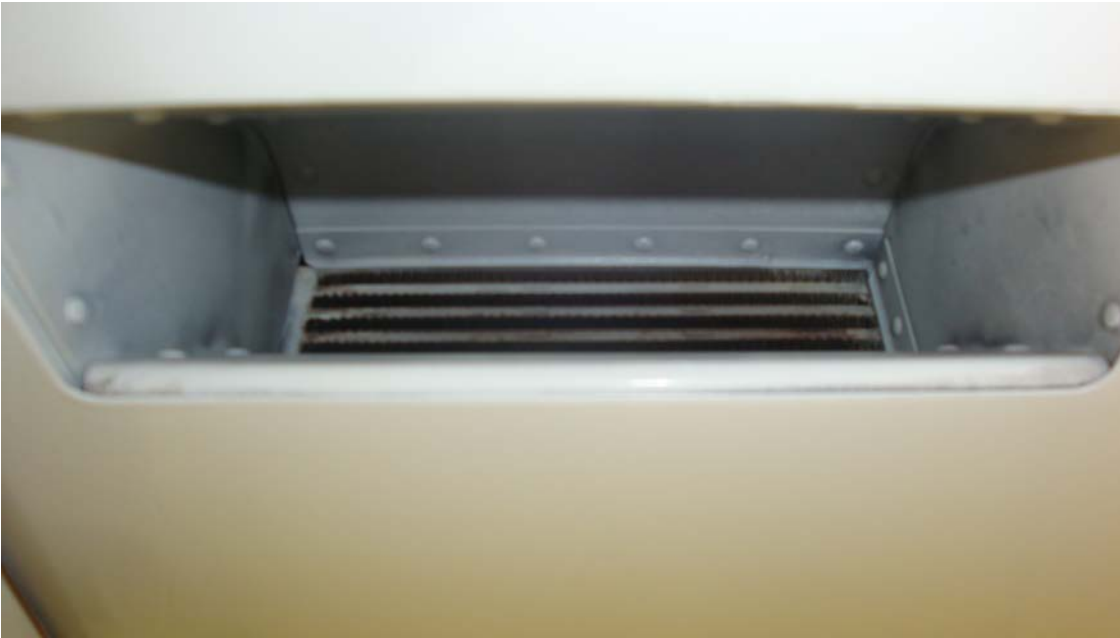
Pylon Heat Exchanger, viewed from underneath
