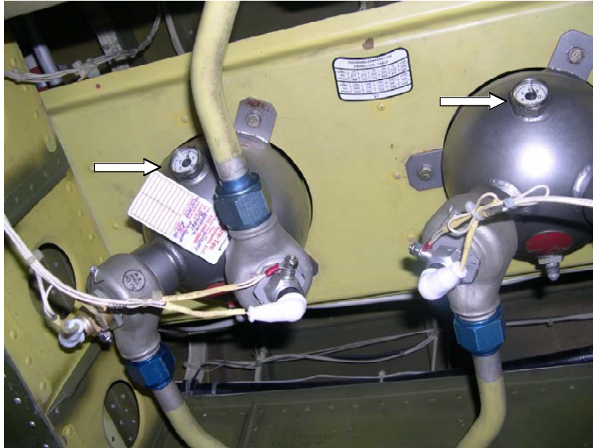
Fire Bottles showing pressure gauges
